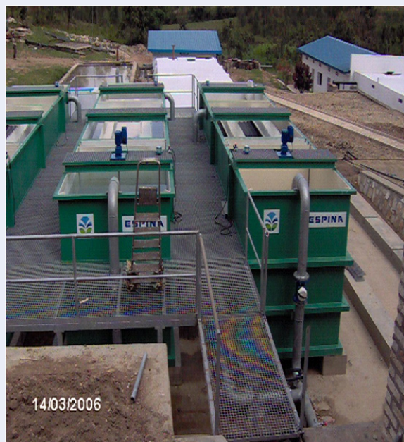
Water treatment plant (Credit: Simon Nduyiye)
