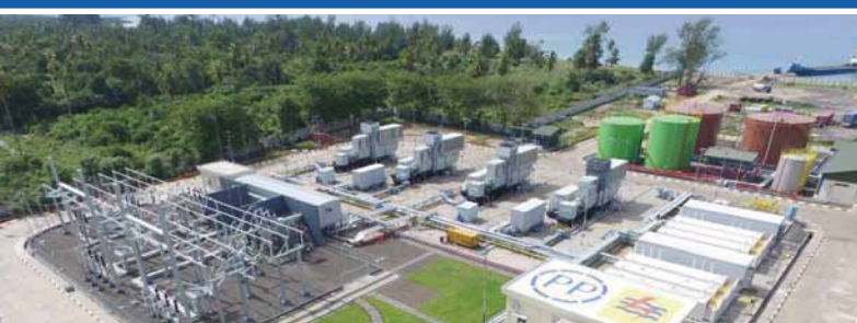
GORONTALO GAS FIRED POWER PLANT PEAKER 100 MW The fastest built power plant in Indonesia
