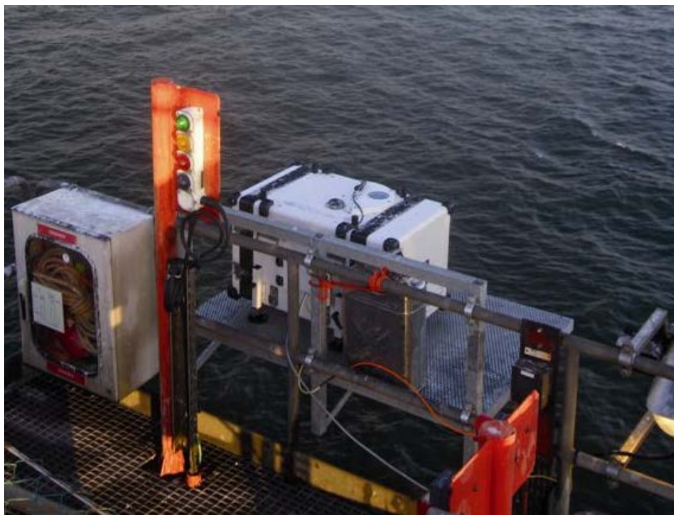
Figure 31: WindCube TM LiDAR on an Offshore Platform. Photo Courtesy of Leosphere
