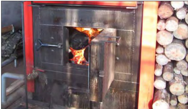
New municipal boiler in Malyn providing heat to three schools, the result of a successful P3DP pilot PPP project.
