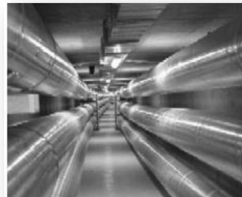
Gas Insulated Lines
