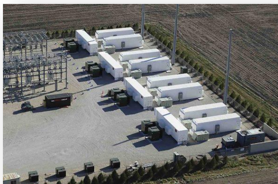
Battery Energy Storage Systems
