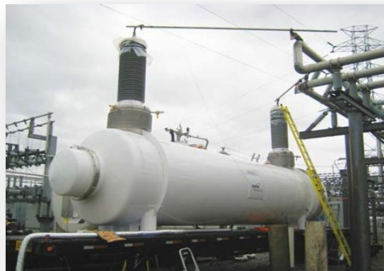
Superconducting Fault Current Limiter
