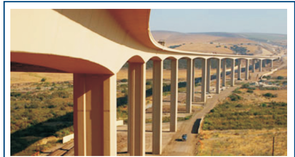
South Bay Expressway, California (DBFO). This 9.3-mile, privately funded toll road was the first PPP to use TIFIA financing (see Glossary). The private franchise—South Bay Expressway, LP—filed for bankruptcy in 2010. (Photo: FHWA)
