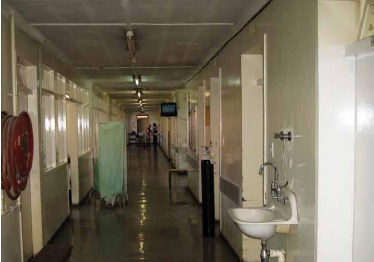
The 100-year-old Queen Elizabeth II Hospital, an aging facility functioning at a minimal level, will be replaced by a new hospital.
