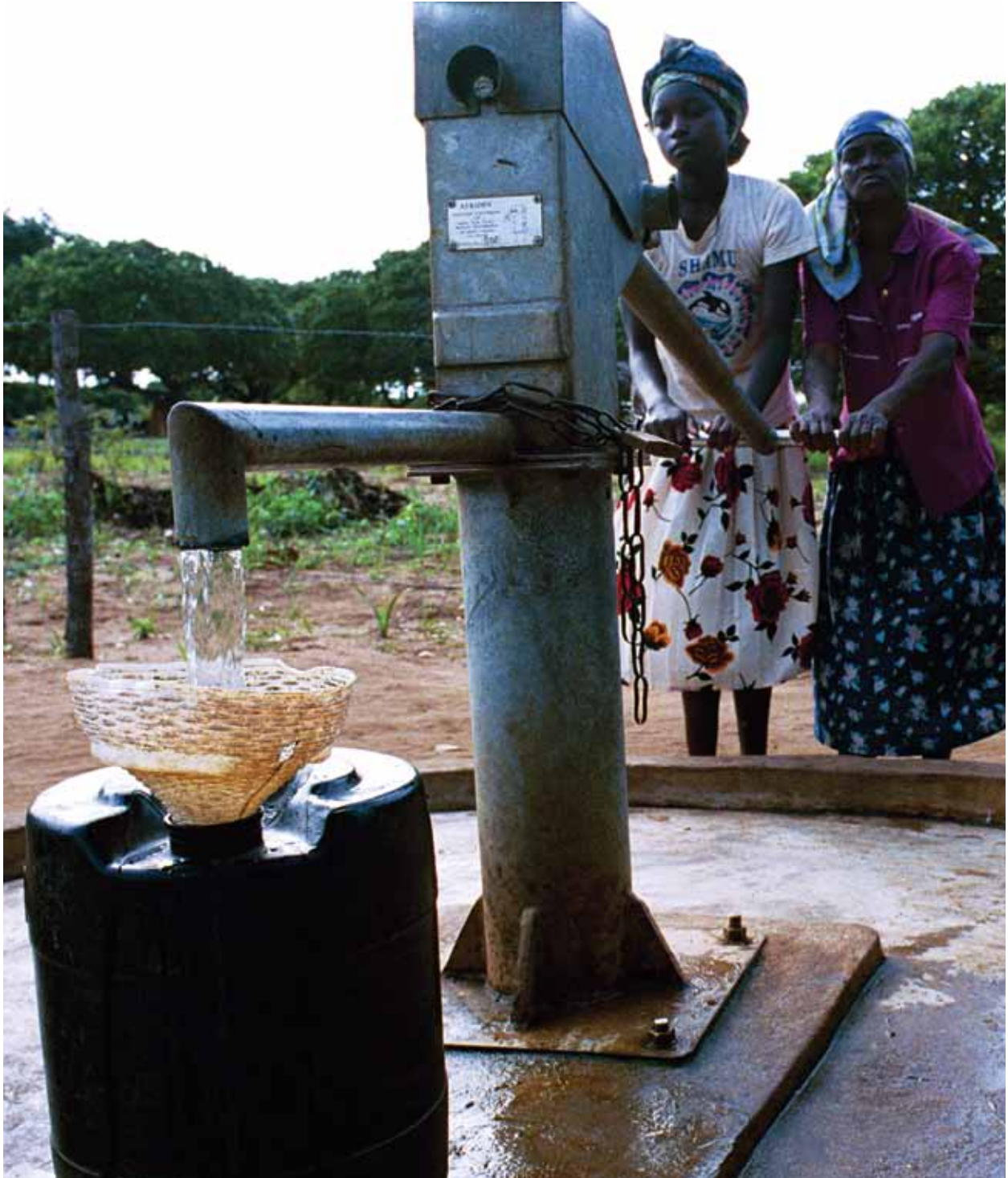
In 2004, Benin constructed more than 1,200 water points. A water point is a borehole with a hand pump that can serve 250 people. Or it may be a small supply system with communal standpipes—the equivalent of many water points.
