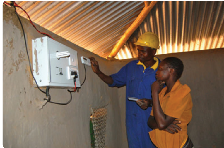
Figure 2. Kenya Power installs prepaid meters, Source: Presentation for the World Bank ( http://cega.berkeley.edu/assets/miscellaneous_files/CEGA_Energy_REPP_June2015.pdf )
