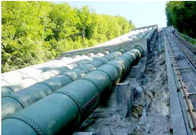
Figure 4-18: Steel penstock of the Walchenseekrafwerk (Germany)
